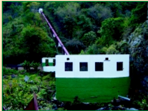
Figure 19: Swaziland Plantations turbine house and penstock
