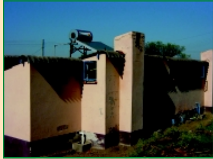
Figure 9: Swaziland Railways solar hot water system
