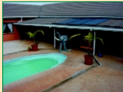
Figure 10: Mr and Mrs Barlow's solar heated swimming pool
